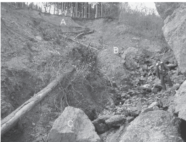
Fig. 4 Close-up photograph of landslide which occurred on July 10, 2002.
